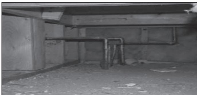
Figure 2. Framed or "platform" return air plenum in an air handler closet in the conditioned space. Plenum had no air barrier, thereby connecting it to the walls and attic, and had dirt, debris, and fiberglass in the space. Photo courtesy Janet McIlvaine and the Building America SM Partnership for Improved Residential Construction.
