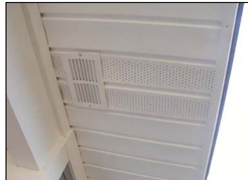
Figure 1: At a minimum, outside air intake register mounted in vented vinyl soffit with outside air duct positioned in soffit above. Note that a filter-back return register is preferred whereas this is a fixed register.
