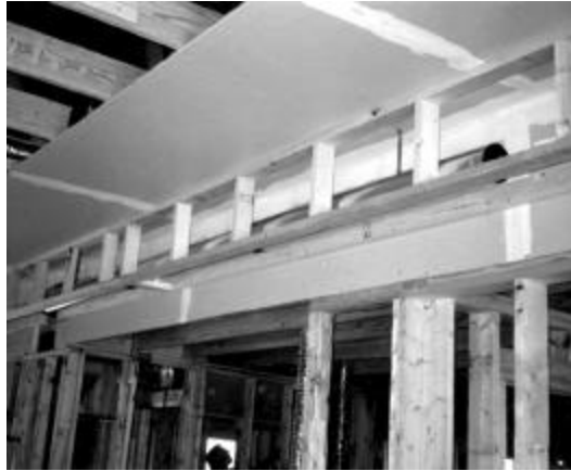
Figure 8 Chase along wall of open living area. Note chase sealing with drywall compound
