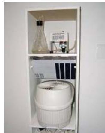
Figure 4 Humidifier, pump and visual indicator
