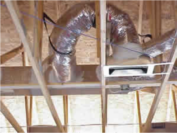
Figure 6. Mastic sealed attic supply duct and plenum.
