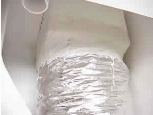
Figure 4. Example of good mastic return connection seal.
