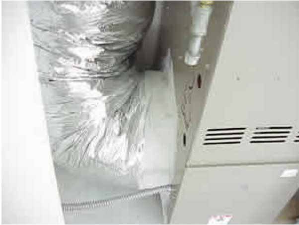
Figure 5. Mastic sealing detail at the air handler return connection.
