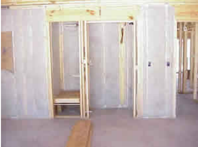
Figure 3. Damp spray cellulose covers walls of mechanical closet (in condition space) and water heater cabinet in the garage. Home entry is on the far right.
