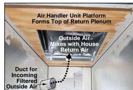
Return plenum with ventilation duct. ~25cfm of outside air enters return plenum when air handler is operating
