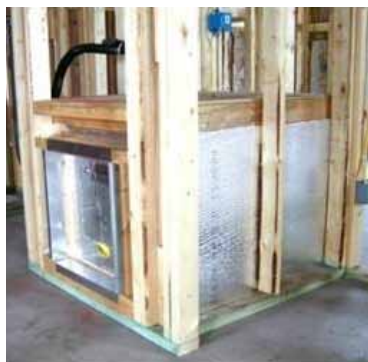
Ducted return plenums ensure that no attic air is accidentally pulled down the wall cavities into the return air stream.
