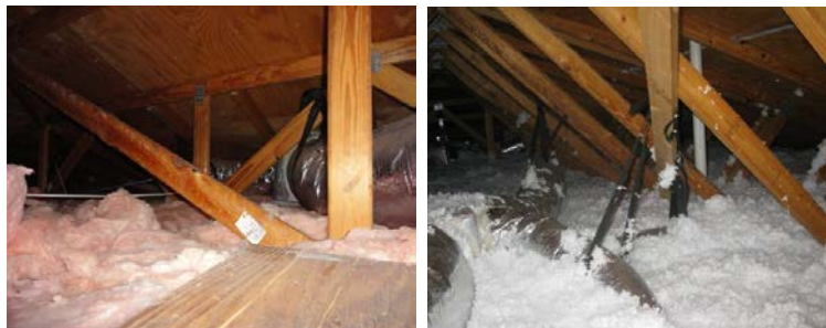
Figures 8-9. Pre-retrofit (left) and post-retrofit (right) ceiling insulation.
