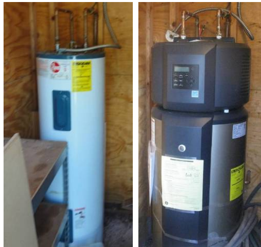
Figures 6-7. Pre-retrofit electric tank water heater, EF = 0.88 (left), hybrid heat pump water heater, COP = 2.35 (right).
