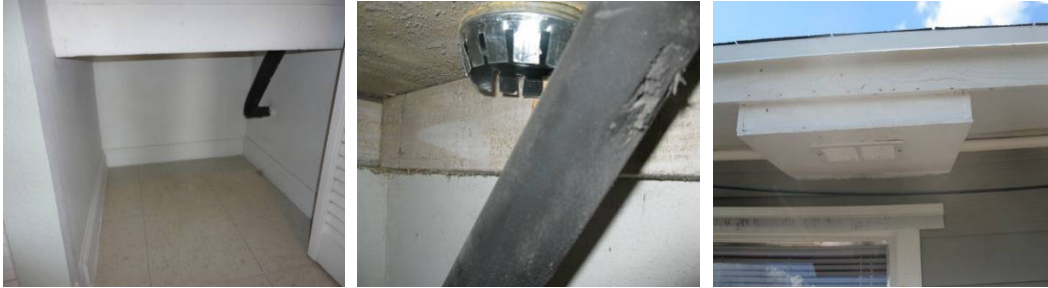
Figures 3-5. Pre-retrofit return plenum (left), outside air ducted into the post-retrofit return plenum (middle), soffit retrofit for the air intake (right).
