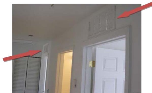
Figure 2. Above door transfer grilles.
