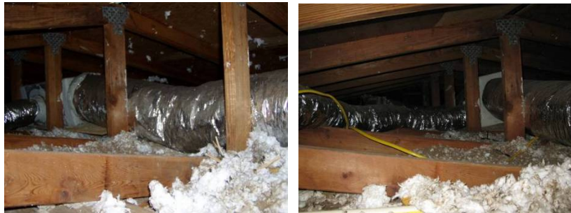
Figures 5-6. Ceiling insulation: Pre-retrofit estimated average of R-11 (left), post-retrofit no additional insulation (right).
