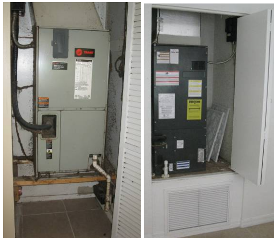
Figures 3-4. Air Handler Closet: Pre-retrofit without return plenum and installed behind airflow-restricting louvered doors (left), Post-retrofit platform return plenum with filter access on same plane as wall (right).
