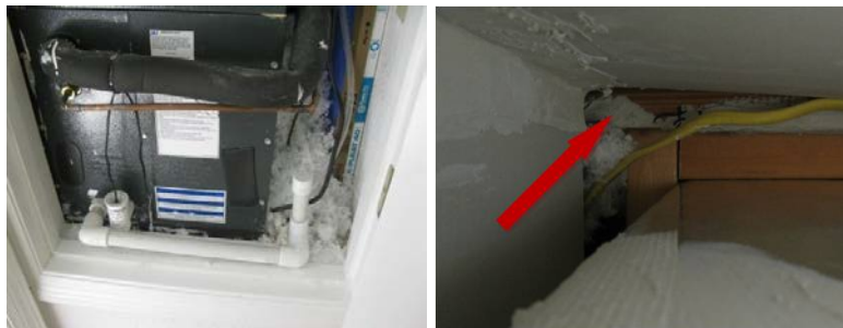
Figures 3-4. White attic insulation around air handler (left) fell through spaces in the closet ceiling (right, looking up at closet ceiling framing).
