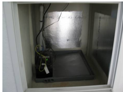
Figure 5. New return air plenum constructed of foil faced duct board, shiny side facing in.
