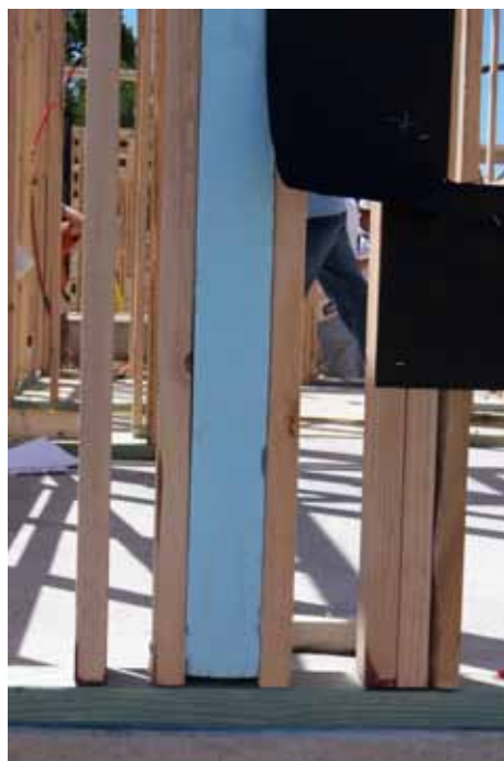
Insulation in corners and interior and exterior wall intersections reduce thermal bridging which can lead to moisture and comfort issues.
