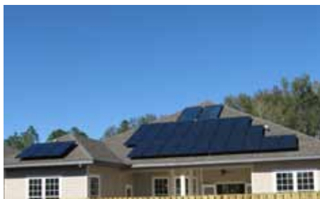
6.75kWp PV system with 64 sq. ft. solar hot water system
