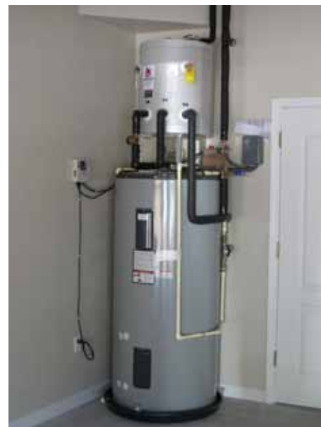
120 gallon storage hot water tank with drain back tank above
