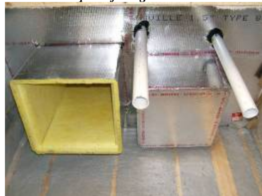
Figure 3-12 Air barrier in top of air handler closet created with duct board by the mechanical contractor at the time that the ducts are installed.
