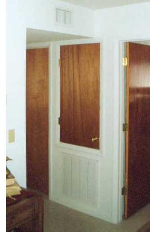
Figure 4-7 An interior air handler, return plenum and supply duct chase
