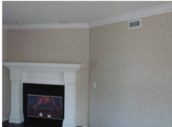
Figure 1-3 Interior view of prototype house with high side discharge outlet
