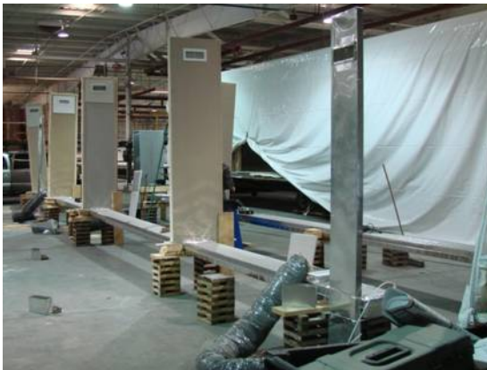
Figure I-3 Floor duct system with high side discharge outlets under construction being tested with duct tester
