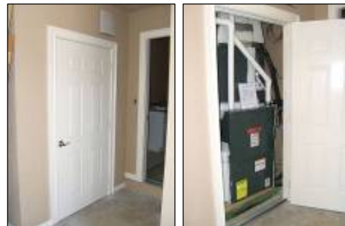
Figure 3-11 Exterior walls around air handler isolate closet from garage, create valuable conditioned square footage.
