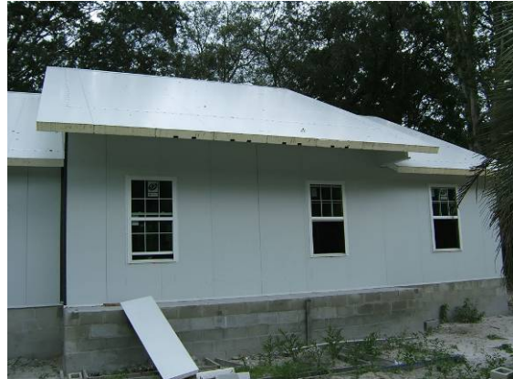
Figure 2-11 Channels in roof construction to allow ventilation of potential heat generated from pv
