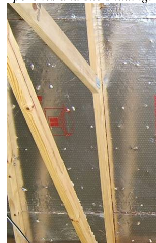
Figure 4-9 Radiant barrier reduces heat transfer from the roof, a major component of the cooling load.
