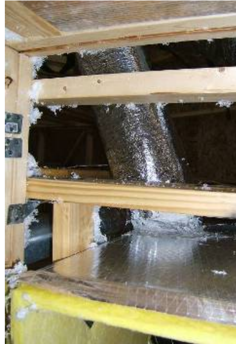
Figure 3-21 Outside air ventilation duct termination into return plenum
