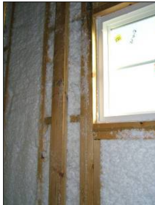
Figure 3-19 Close up of ladder detail at the intersection of an interior wall. “Rungs” provide drywall nailing surface without compromising insulation.
