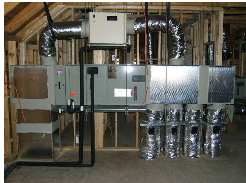
Figure 2-4 HVAC equipment installed
