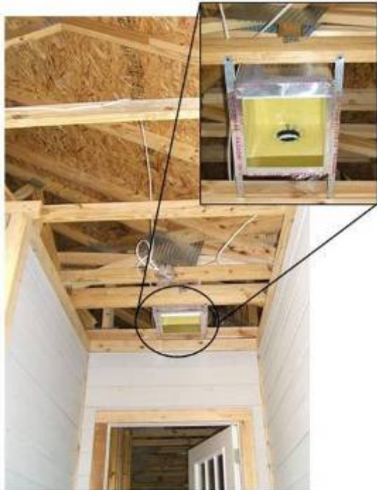
Figure 3-20 Outside air intake boot in porch ceiling at front door
